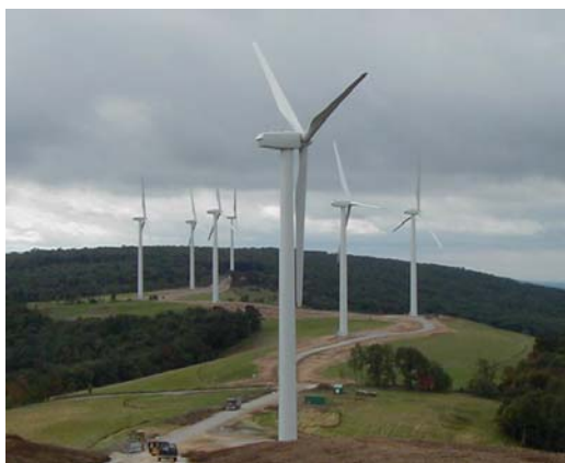
The 15-MW Mill Run Wind Farm On-Line October 2001
