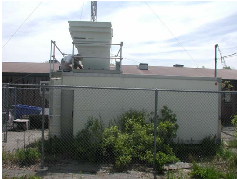
Figure 3. Close-up of the SODAR on the building.
